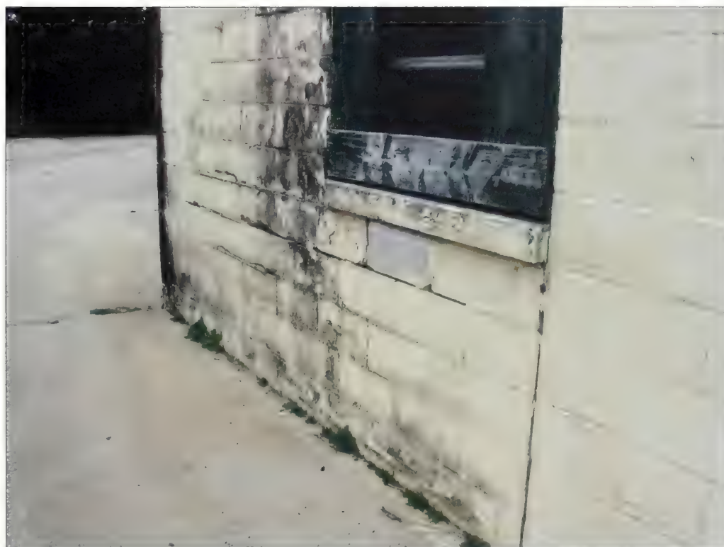
Figure 5.121. View looking northwest at Warhead Building (450), NIKE launch site. Routine maintenance procedures will help stabilize free-standing buildings in the launch site. The water damage seen in this image originates from a metal gutter mounted at the top of the wall that needs to be cleaned and reset so water is carried away from the building (Olmsted Center, April 2008).
